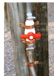
drip irrigation valve from cistern
